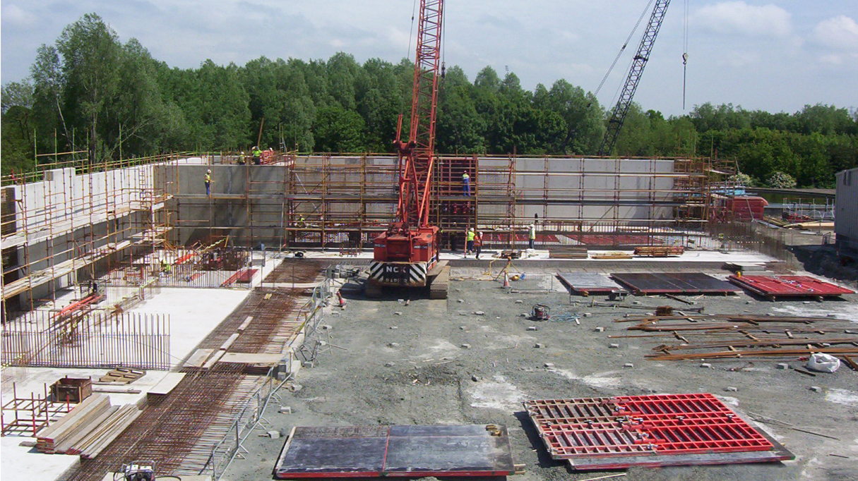
Improvements at Stirling Waste Water Treatment Works to provide capacity for growth.
