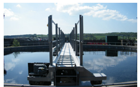
Carbarns Water Treatment Works
