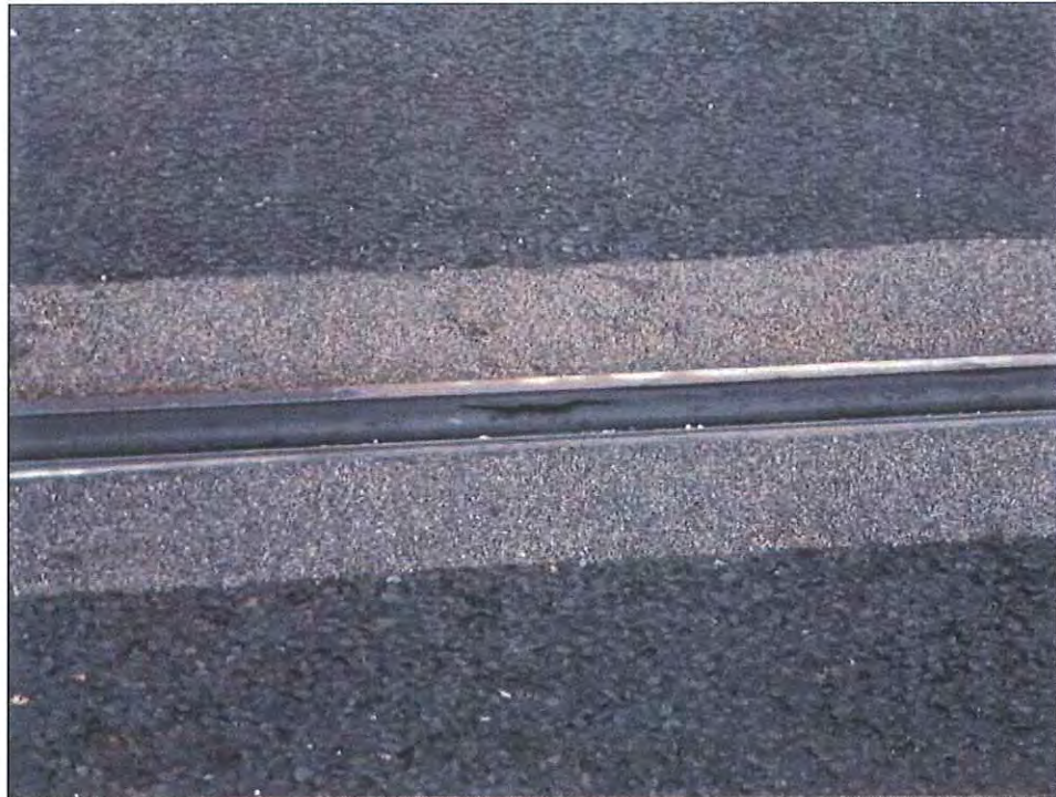
Figure 2.1 – Joint Seal Tear
