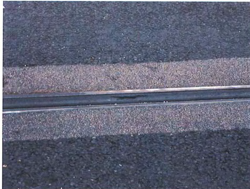
Figure 6: Tear on Eastern Joint Seal
