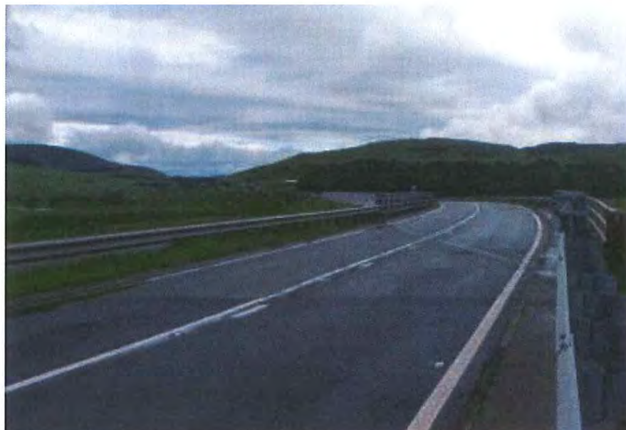
Figure 4: Looking North East across the structure, from the western end of the southbound carriageway.
