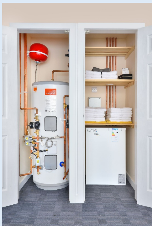
Figure 11: Image of Cupboard Comparison showing space saving using water cylinder. Provided by Sunamp (January 2021)
